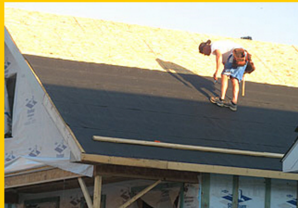
Roof work at Habitat for Humanity Summer 2009 Build Site. Photo: Katy Mike Smaistrila.
